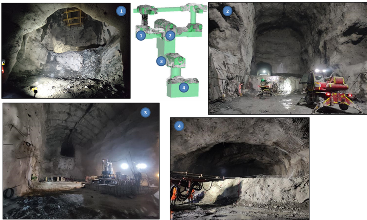
Figure 8 Ground control inspections during intermediate construction stage for different caverns and large excavations (Valdivia & Parada 2020)
